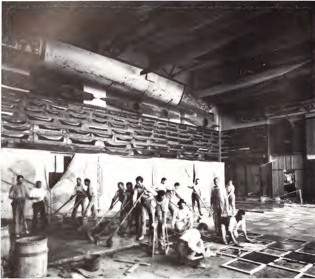
Cement floor being put in at the United States National Museum, with Pacific Northwest Indian canoes hanging above. This was probably taken in the late 1880s to 1890 after the original wooden floor rotted away.
